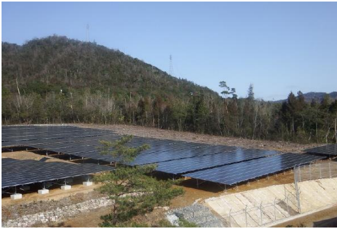
Higashi-Hiroshima Mega Solar Power Plant (Hiroshima Prf., 1,000 kW)
