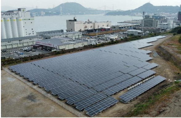
Mojikazashi Solar Power Plant (Fukuoka Prf., 1,400 kW)
